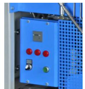
Semi automatic compressor control
